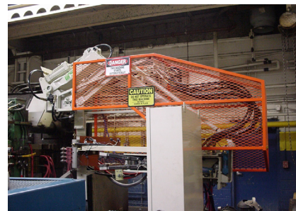
New Rimrock extractor installed on #41 zinc die casting machine
